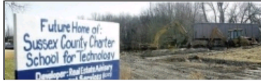
Photo by Amy Paterson/New Jersey Herald Work continues at the site of the new $5.2 million Sussex Charter School.
